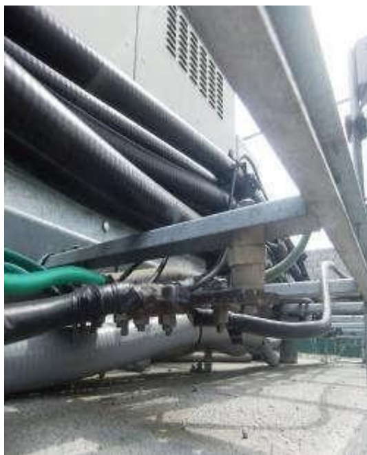
Figura 36. Barra de tierra Outdoor
